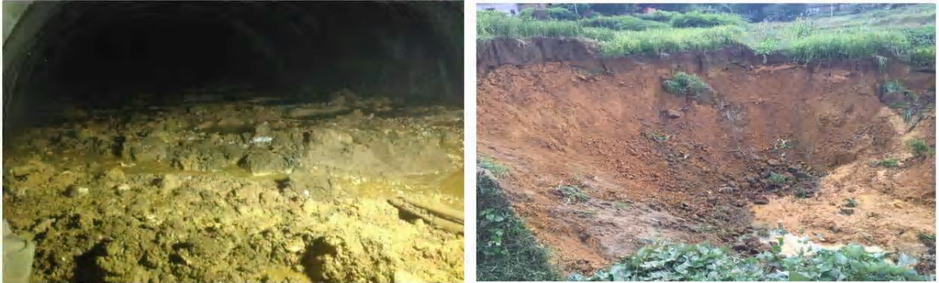
Figure 6 Surface collapse of Tu Ni Yao.
