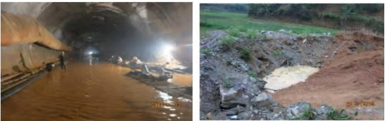
Figure 5 Surface collapse situation of sudden mud and water gushing Yao.
