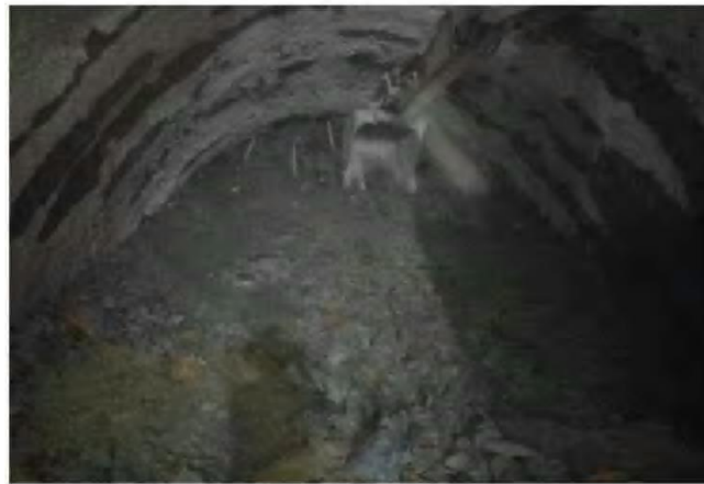
Figure 2 Barrow II tunnel slip and fall site figure.
