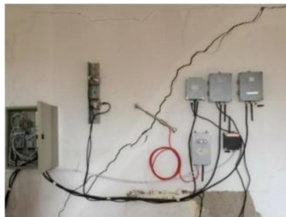
Figure 2 Acceleration sensors and seam gauges.
