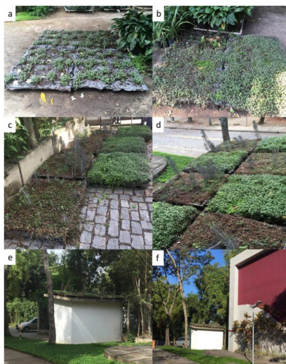
Figure 1. Stages of the green roof assemblage (a) initial planting of succulents on the pallets after the geotextile coverage; (b) development of the vegetation; (c) pallets positioning before the assemblage on the rooftop; (d) green roof modules after the placement on the rooftop; (e, f) external view of the green roof.
