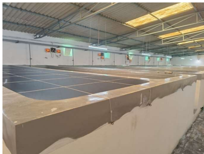
Figure 2. Automation devices installed in the hatcheries.
