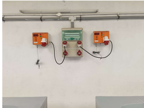
Figure 3. A closer view of the installed device.
