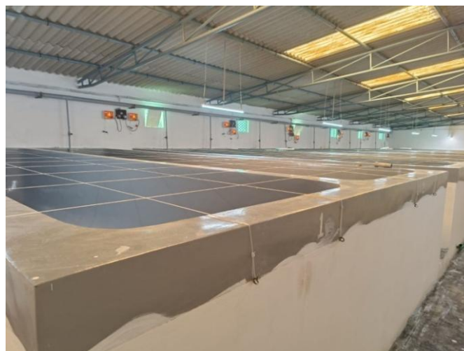
Figure 2. Automation devices installed in the hatcheries.
